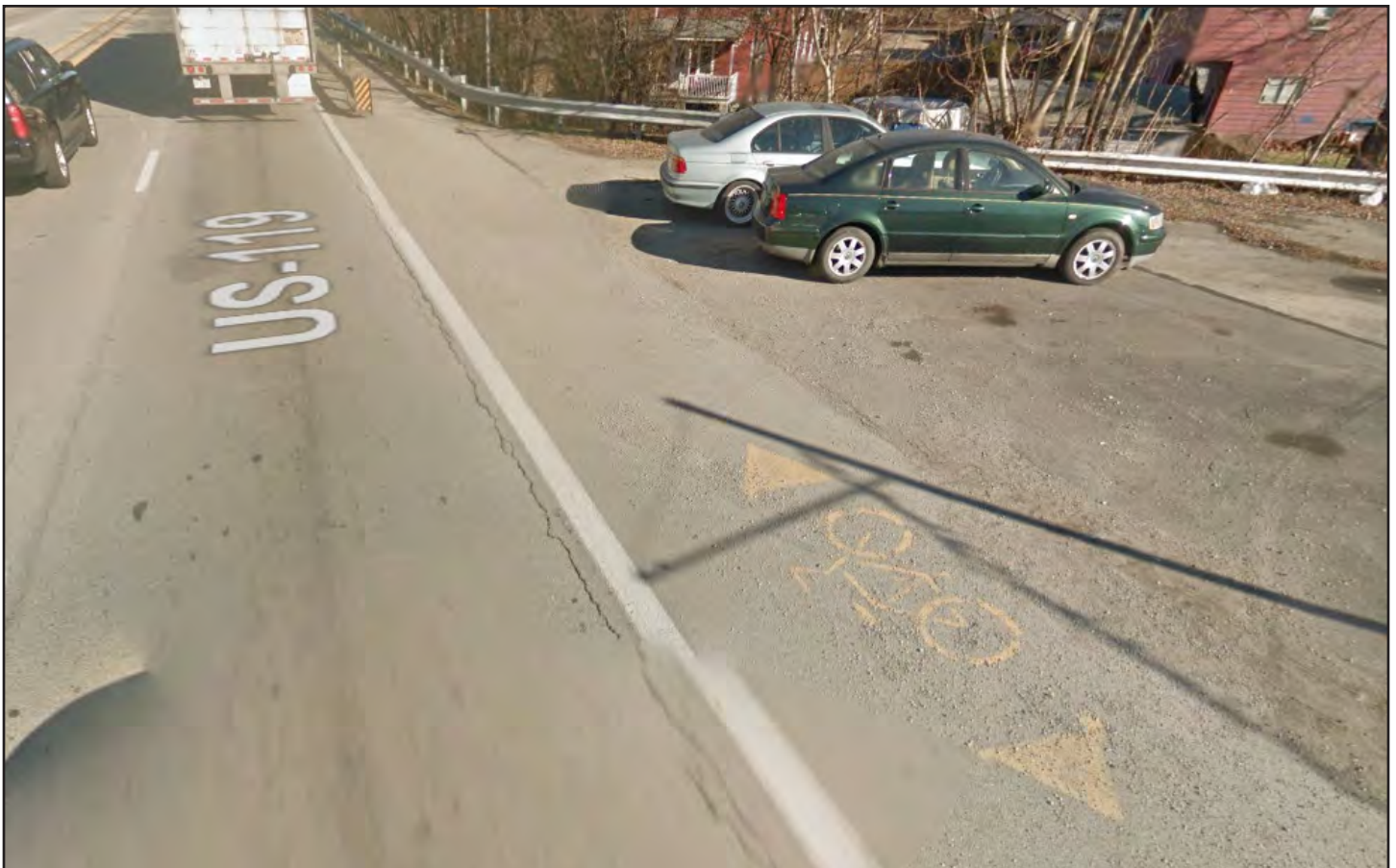
A gravelly shoulder along Route 119, which has a posted speed limit of 35 mph, makes for an uninviting route from 7th Street to Memorial Bridge..
